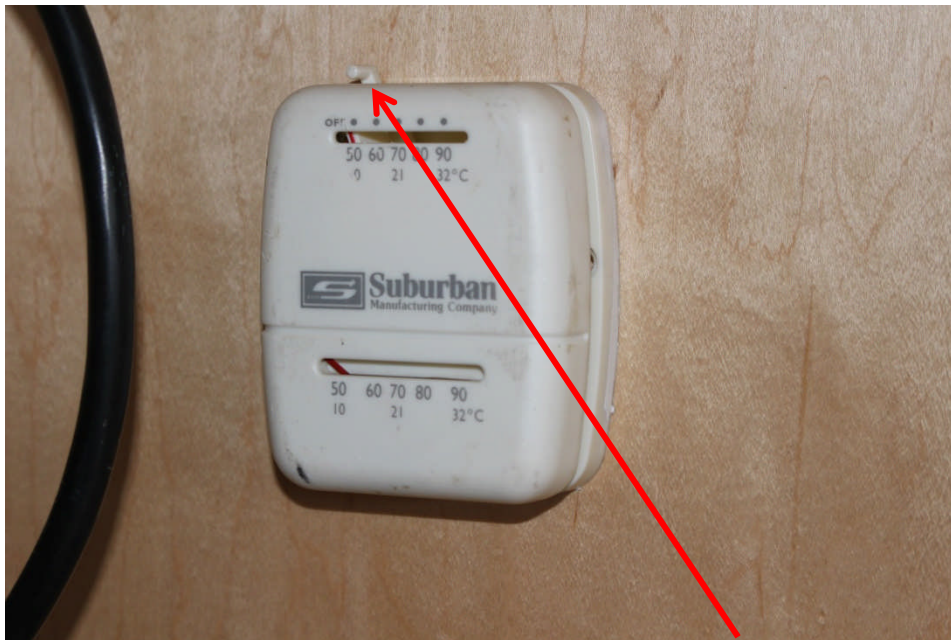
Turn Thermostat off, lowest temperature
