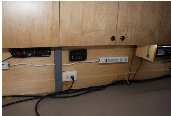
DC, AC PWR, INVERTER CTRL ANT & PUSHUP MAST STORAGE
